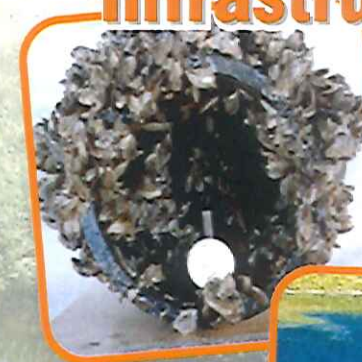
Quagga mussel growth on ABS pipe from Lake Mead, Arizona
