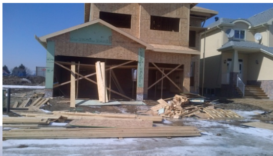
Construction materials / debris on street / boulevard / sidewalk (left)
