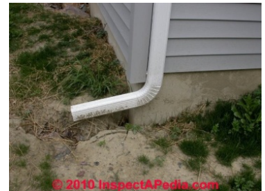
Figure 3 – Erosion occurring from unprotected drainage of downspout (Source: http://inspectapedia.com/ )
